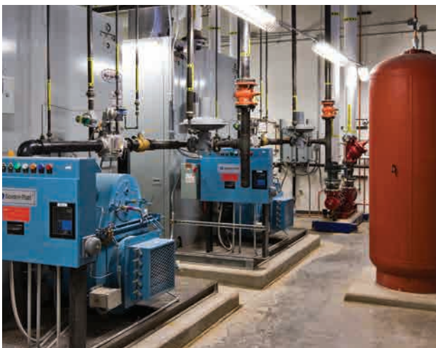
Bottom Left: High-efficiency hot water boilers
