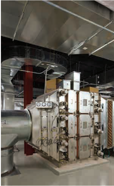
Above: HEPA filter plenum for efficient cooling of clean rooms
